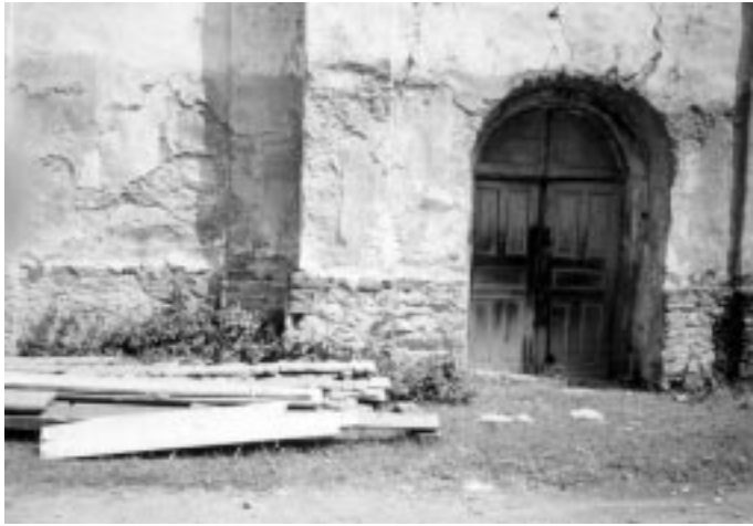
Church in Nyzhniy Bystry in need of restoration.
